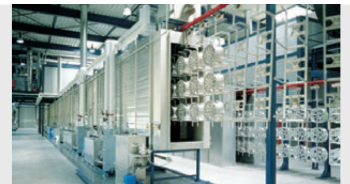
Pretreatment plant for chromium-free conversion treatment.
