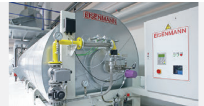
Eisenmann exhaust air purification.
